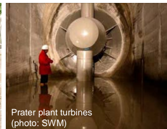
Invisible power plant under the river (photo: SWM/Green City Energy)
